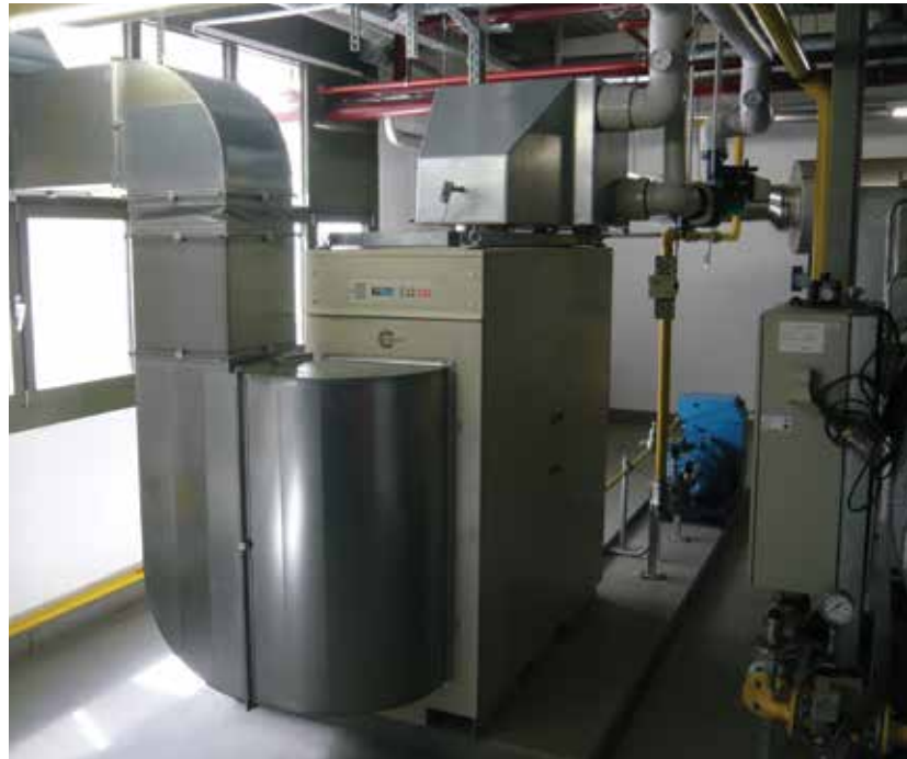
The Capstone C65 cogeneration system saves the hospital €22,500 annually in energy costs.
